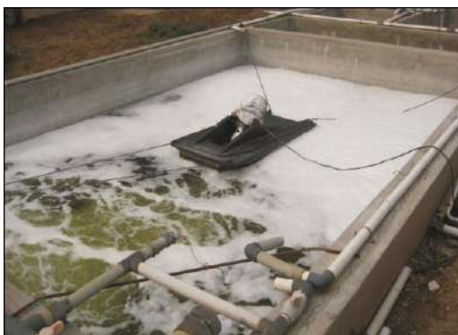
Recycling Waste Water Treatment Plant
